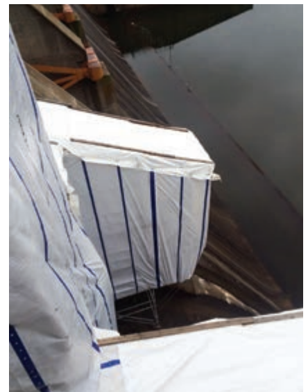
FIG. 7: Containment and scaffolding structures were constructed around tainter gates during the project.
