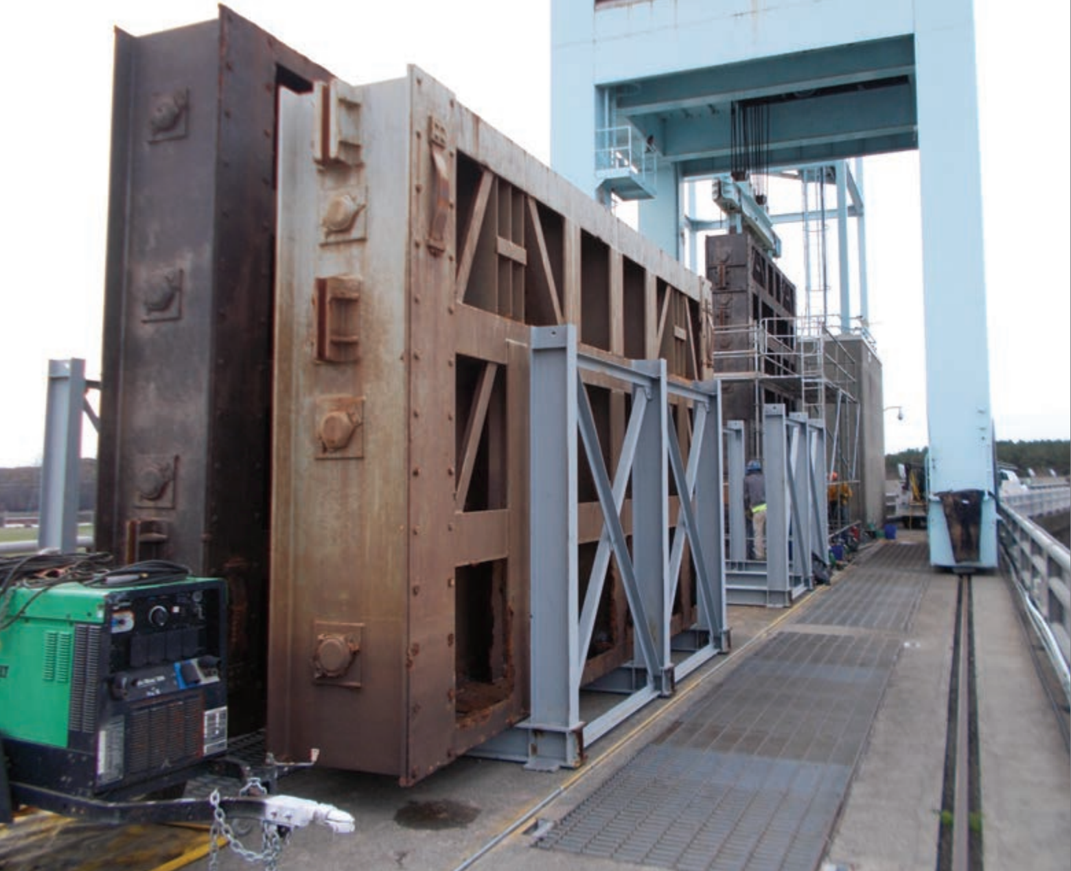
FIG. 2: Intake pieces were disassembled before being transported by crane to an onsite building for repairs, blasting and coating.
