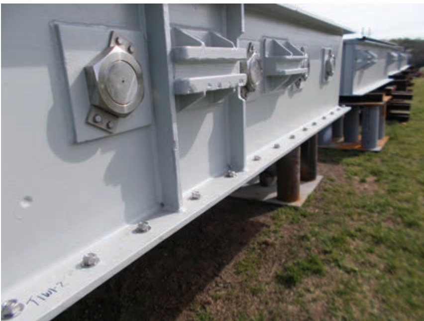
FIG. 4: Intake and tailrace pieces received two stripe coats and three full coats of a polyamide epoxy coating.
