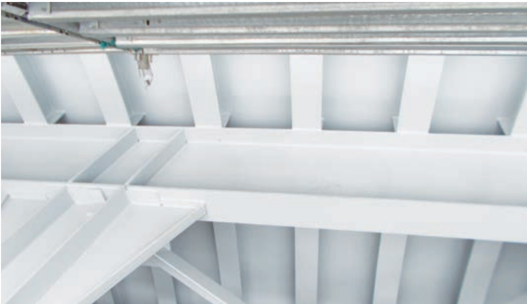
FIG. 8: The downstream sides of the tainter gates received an additional coating of epoxy and an acrylic polyurethane finish coat.
